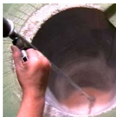
The assembly opening is to fill with special hole mix and to vibrate.
